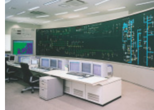
Power-system monitoring control system
