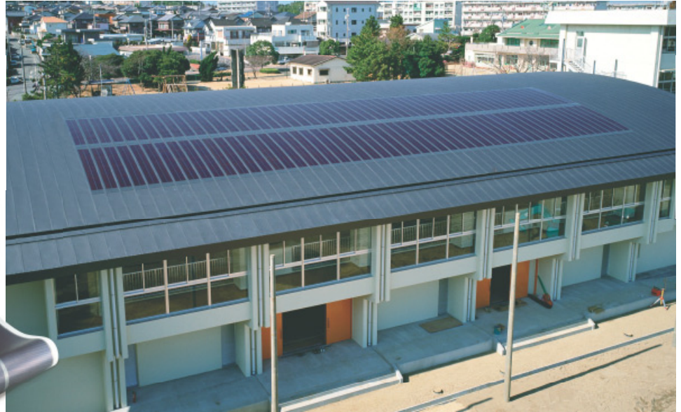
Photovoltaic power generation systems
