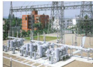
Extra high-voltage substation equipment
