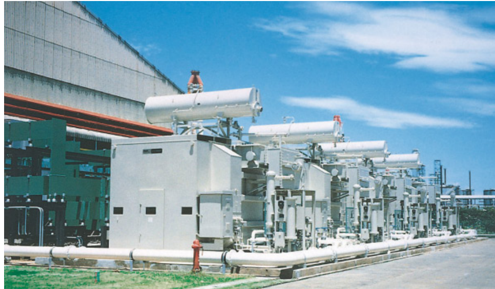
High-capacity rectification equipment
